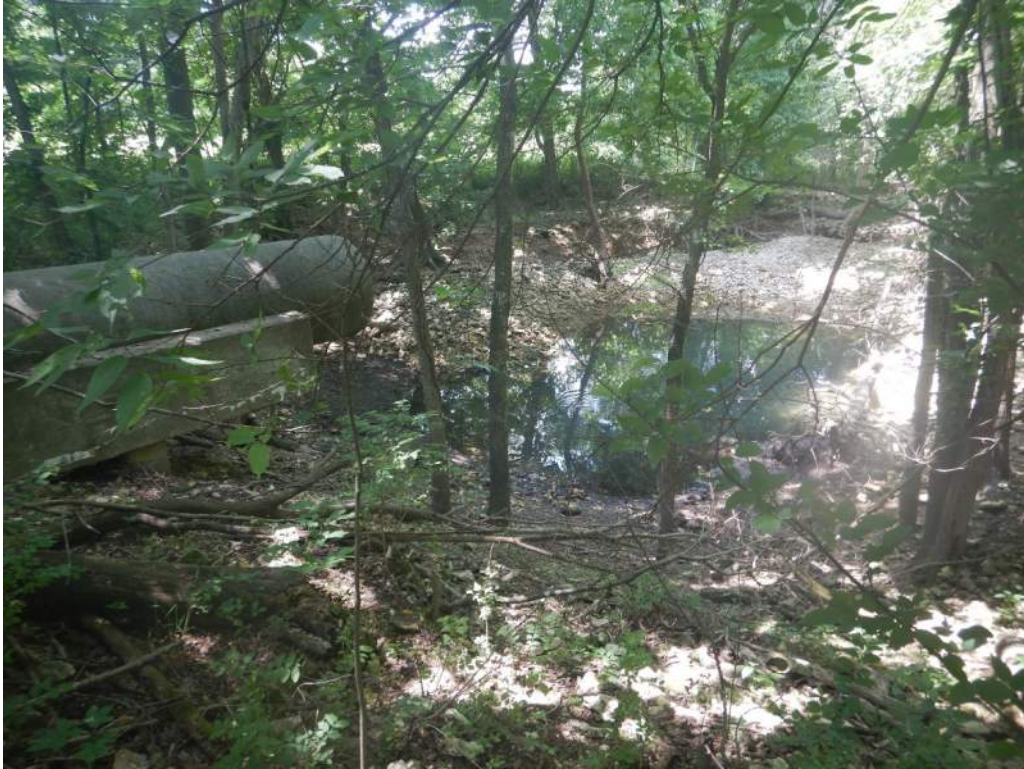
Photo 3. View looking north (downstream) along Stream 1 and the principal spillway outfall north of the Scaper Hollow 2 FRS.
